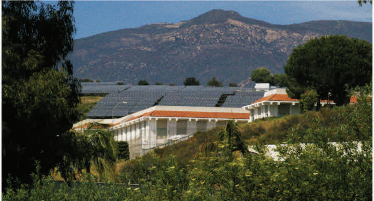
A $5.2 million array of solar panels sits on the hillside behind the Santa Barbara County Jail, part of the county's effort to reduce its carbon footprint and energy costs. (Tom Bolton / Noozhawk photo)
