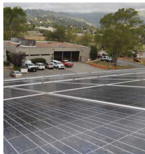
Ground mounted solar panels behind Mill Valley’s Public Safety Building
