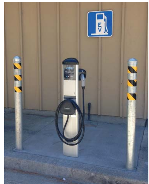
Electric vehicle charging station near Hauke Park
