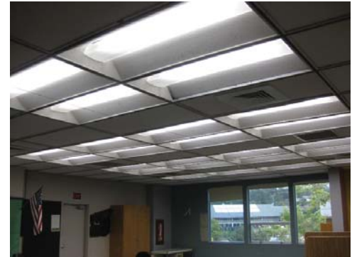
New lighting at Mill Valley Middle School
