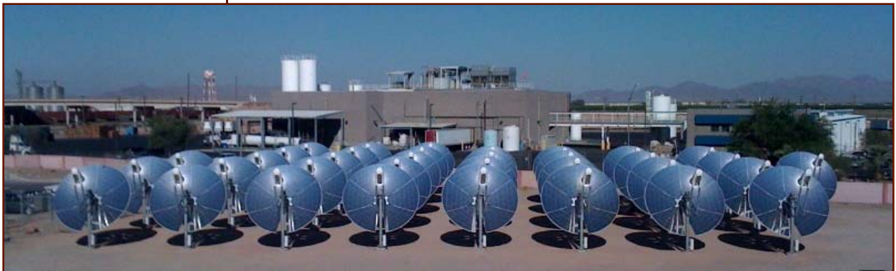
The City of Tulare is installing a solar dish plant at the wastewater treatment plant
