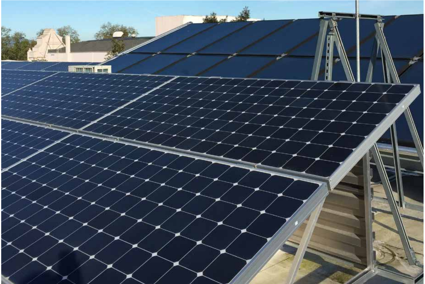
Solar panel array on the rooftop of the Zero Net Energy West Branch Berkeley Public Library
