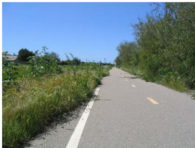
Photo 27: Neglected bike path in Lompoc Valley
