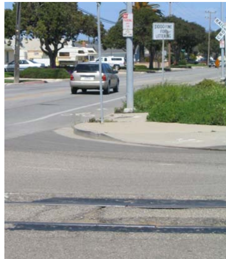
Photo 16b: The City of Lompoc has filled in the gaps between these rail road tracks on Laurel Ave. with paved tapered approaches. Another retrofit for railroad crossings is rubberized strips that decrease the gap and keep the crossing smooth for bicycles and cars alike (Photo 16a)..
