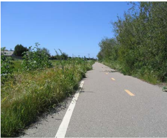
Photo 3: This Class I facility in the City of Lompoc connects the residential western half of the City to the commercial centers along Highway 1. Note the need for brush clearing (maintenance issues covered in Chapter 3).
