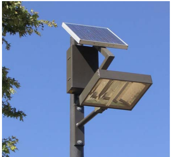
Photo 15: Solar lights were installed on the Obern Trail in Santa Barbara to increase bikeway visibility and safety for commuters in the evening hours. Photo courtesy of Ralph Fertig
