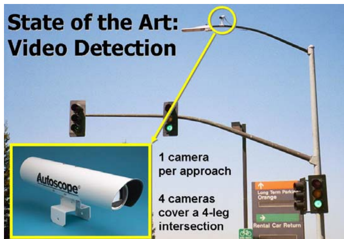
Photo 19: State of the Art Modern Video Detector/Sensor, most common in busy intersections
