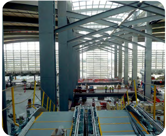
The new International Terminal B at the Sacramento International Airport (shown here under construction in 2010) was designed with green building features to achieve LEED certification. (Photo: SCAS)
