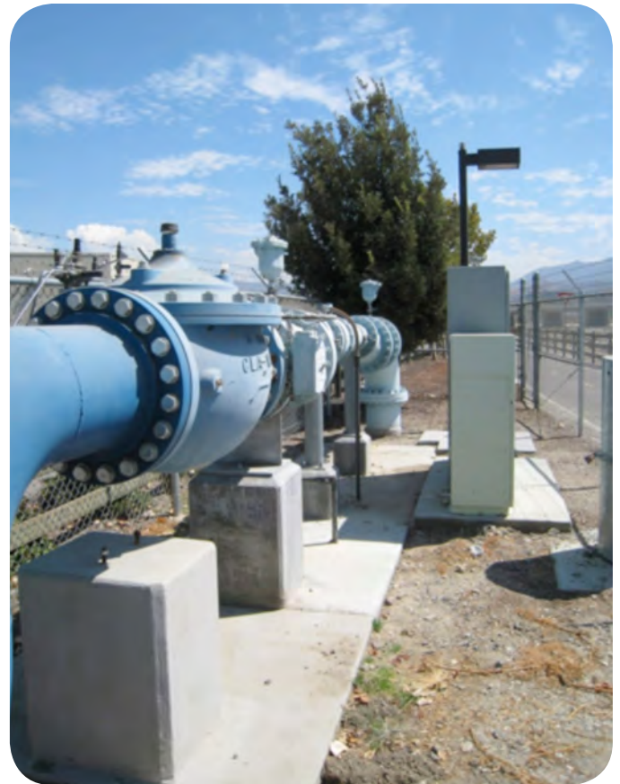
Groundwater pumping and distribution systems are energy intensive and strategies for future operation should focus on maximizing efficiencies and ensuring reliable supplies in the face of an uncertain climatic future. (Photo: www.aquaforia.org )
