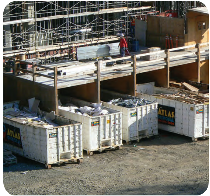
Existing regulations require contractors to recycle 50% of construction and demolition debris (Photo: County DWMR)
