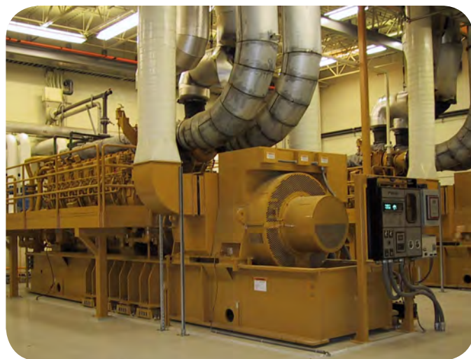
The Kiefer Landfill is home to a gas-to-energy plant that collects landfill gases to convert into energy for SMUD to power close to 9,000 homes. (Photo: DWMR)
