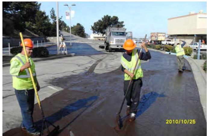
Road reconstruction (top photo) due to deferred maintenance is more energy intensive than slurry seal applications (bottom photo) and other pavement preservation techniques.
