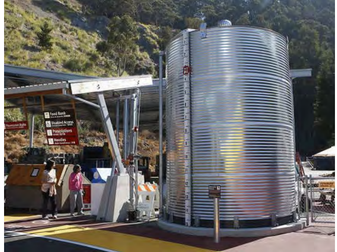
This 11,000 gallon rainwater cistern at the Recycling + Environmental Resource Center offsets use of potable water by using rainwater for toilet flushing and irrigation.
