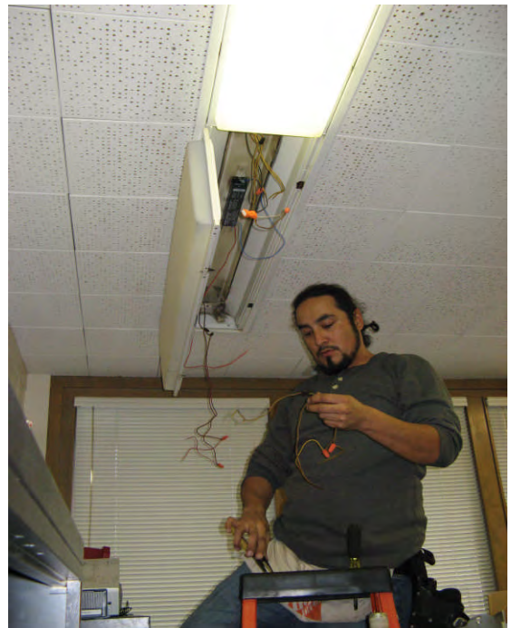
In a business, lighting efficiency upgrades are some of the most cost-effective ways to save energy and reduce costs.
